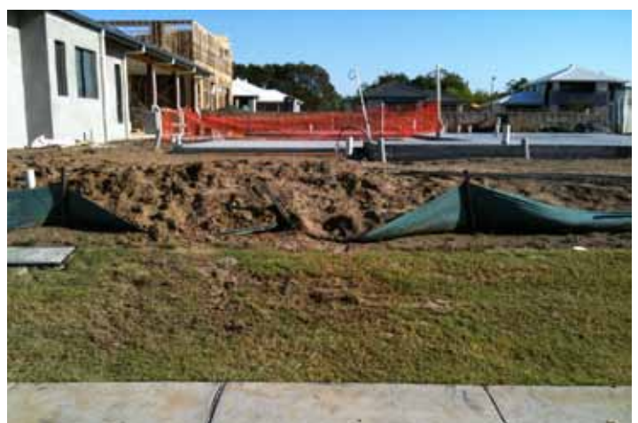
Failed sediment fence with sediment trapped in turf downhill (top)
